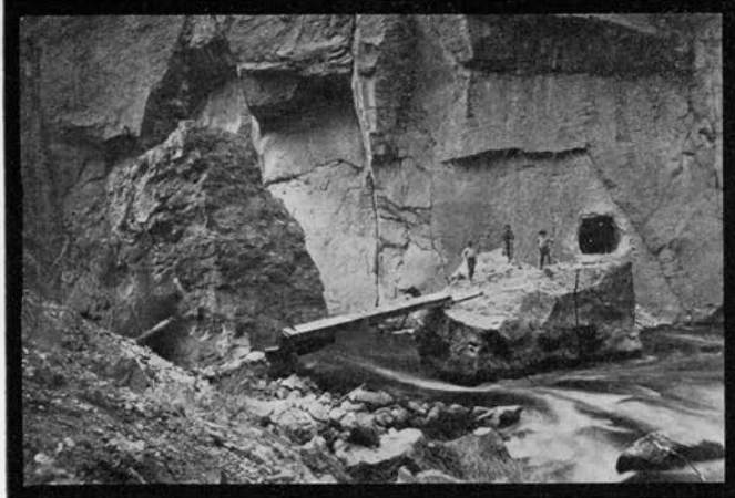
Upper Intake of Mono Power Co. showing upper mouth of 8000-foot tunnel. A huge dam is being constructed just below the big rock in the foreground of the picture.
